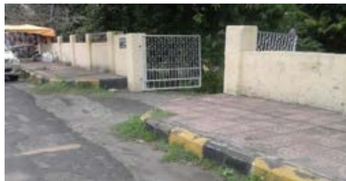
Figure 40 - Pedestrian path's high and low cuts cause discomfort to persons with disability
